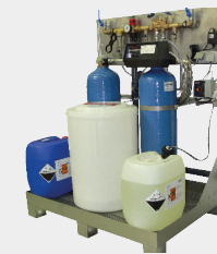
Water treatment systems
